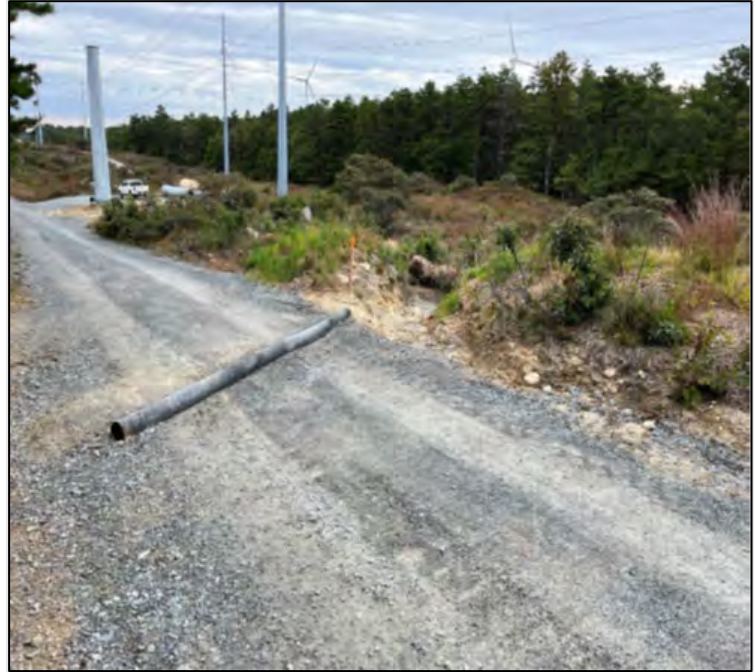
A water bar used to divert stormwater to a plunge pool controls sedimentation and reduces the risk of roads washing out.
