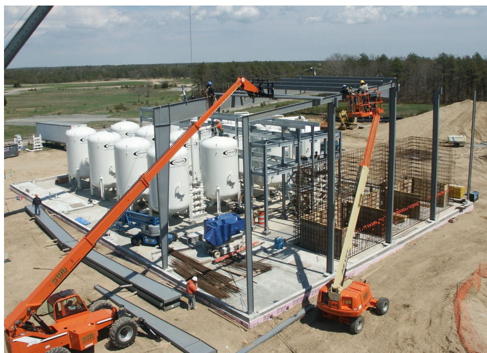
Construction of the Air Force’s largest groundwater treatment facility on JBCC with 16 vessels each containing 20,000 pounds of GAC. The cleanup system treats contaminated groundwater that comes from several plumes on and off-base including CS-21 via extraction wells and pipelines. Cleaned water is then returned to the groundwater aquifer.
